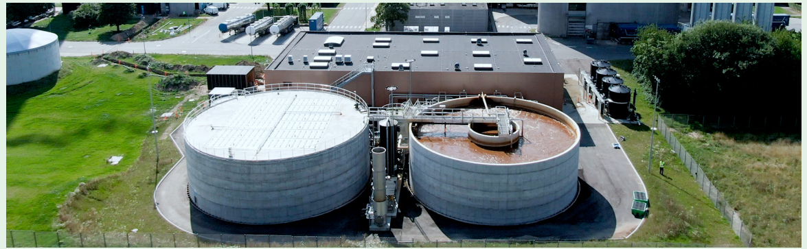
Carlsberg’s Total Water Management plant in Fredericia, Denmark uses anaerobic and aerobic wastewater treatment. The anaerobic tank on the left produces biogas, which Carlsberg uses to produce heat for the brewing processes, adding another layer of sustainability to the project.
